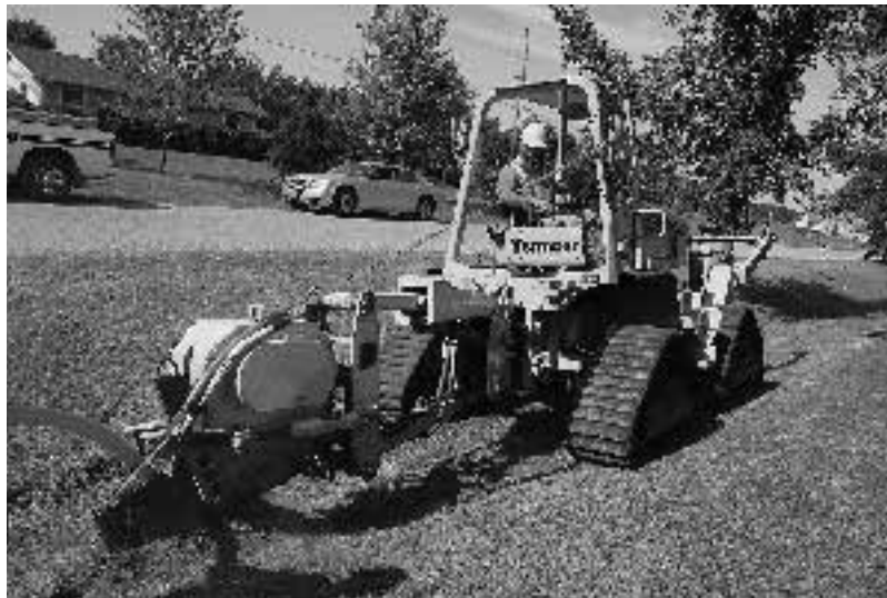
Fig. 2.47 A cable plowing machine that is used in a nonurban environment. (Photo courtesy of © VERMEER CORPORATION. All Rights Reserved; www.vermeer.com .)
