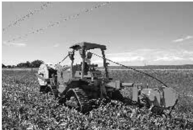
Fig. 1.12 Plowing operation for direct burial of optical fiber cables. (Photo © VERMEER CORPORATION. All Rights Reserved; www.vermeer.com .)
