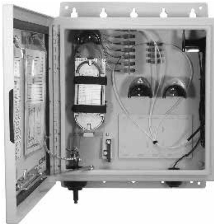
Fig. 13.43 A compact, rugged outdoor cabinet used to interface a multiple-fiber PON cable to multiple indoor ONTs. (Photo courtesy of Charles Industries; www.charlesindustries.com .)
